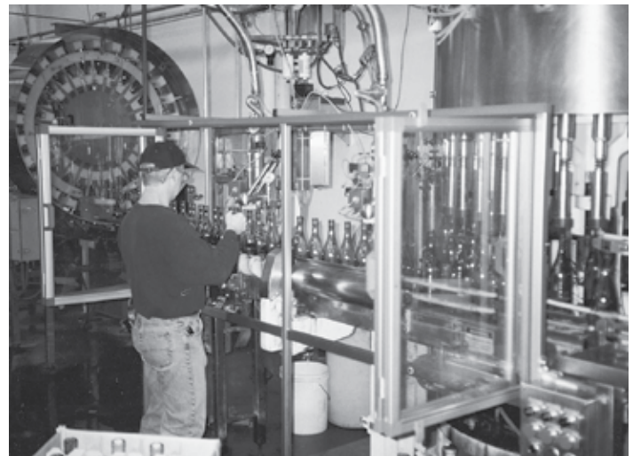
Bifold doors on this free standing enclosure provide easy and unobstructed access to this bottling line.
